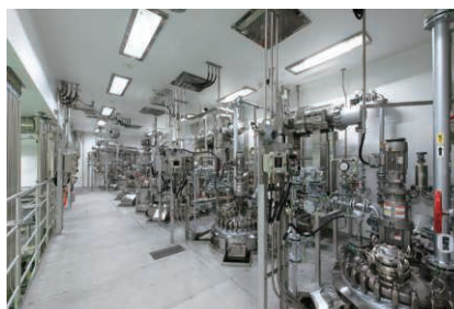
Pharmaceuticals: Manufacturing facility for highly potent active pharmaceutical ingredients
